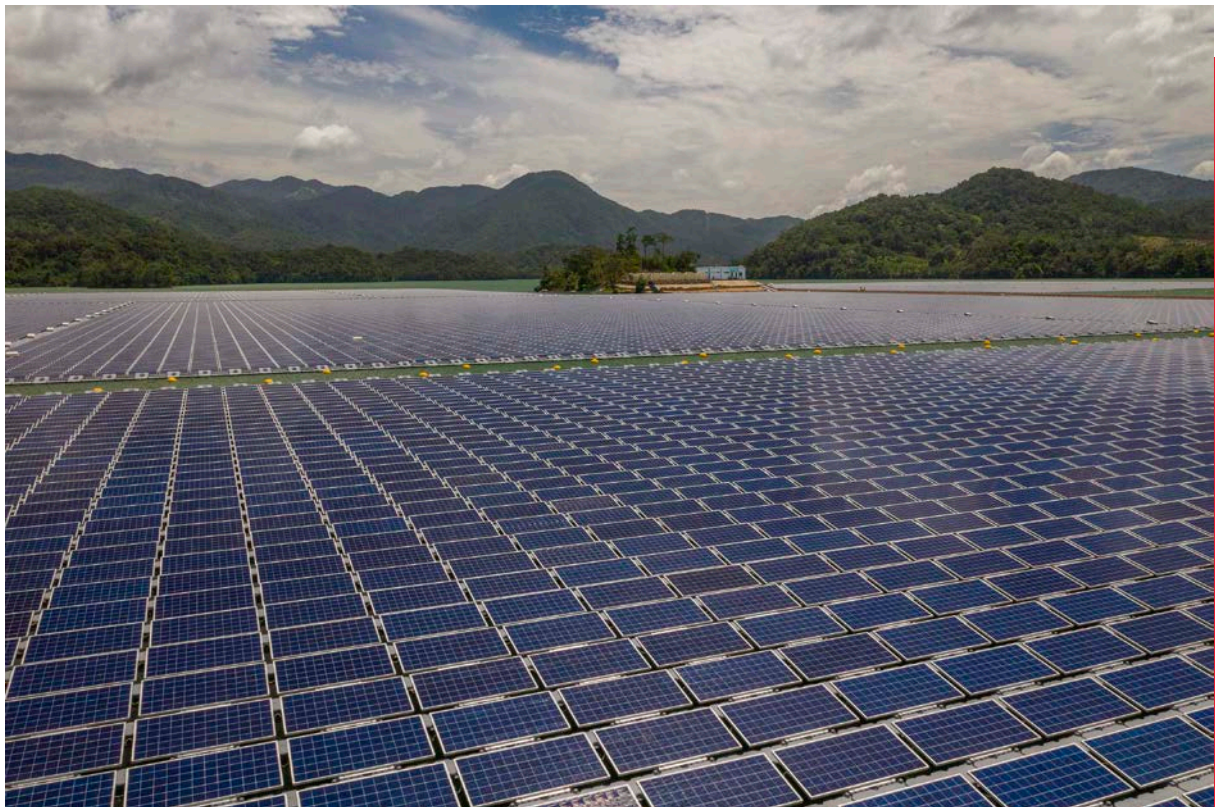
Floating Solar Energy Project in Vietnam. (Image: Asian Development Bank)
