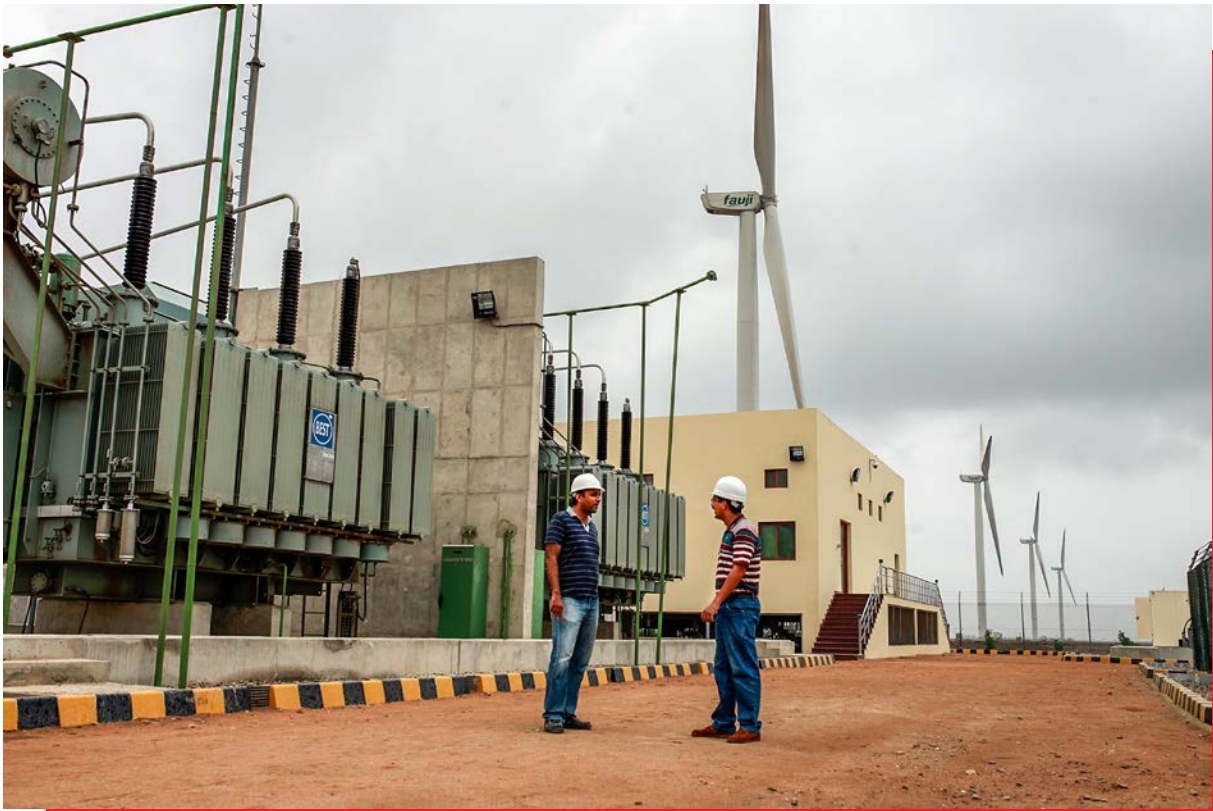
Foundation wind energy in Pakistan. (Image: Asian Development Bank)
